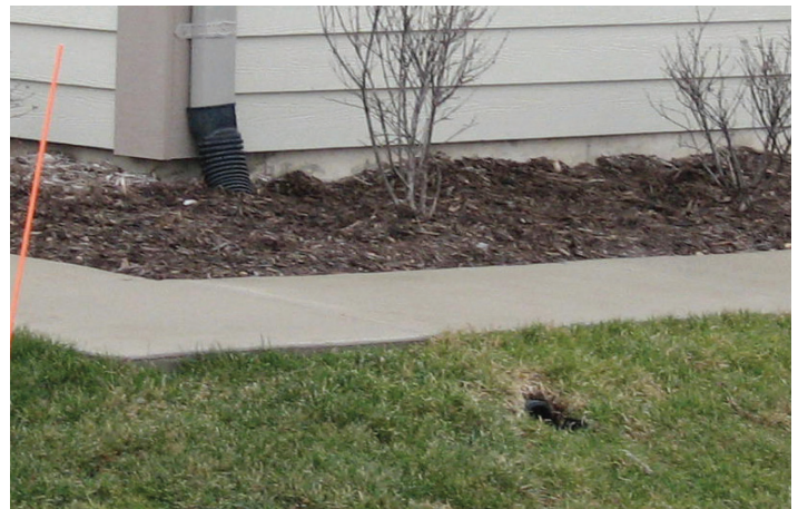
The drain slopes away from the foundation and terminates at the proper distance
