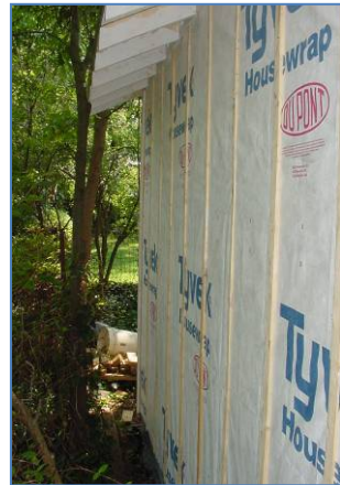
5. If siding is installed in a rain screen configuration install furring strips attached directly to the underlying framing.
